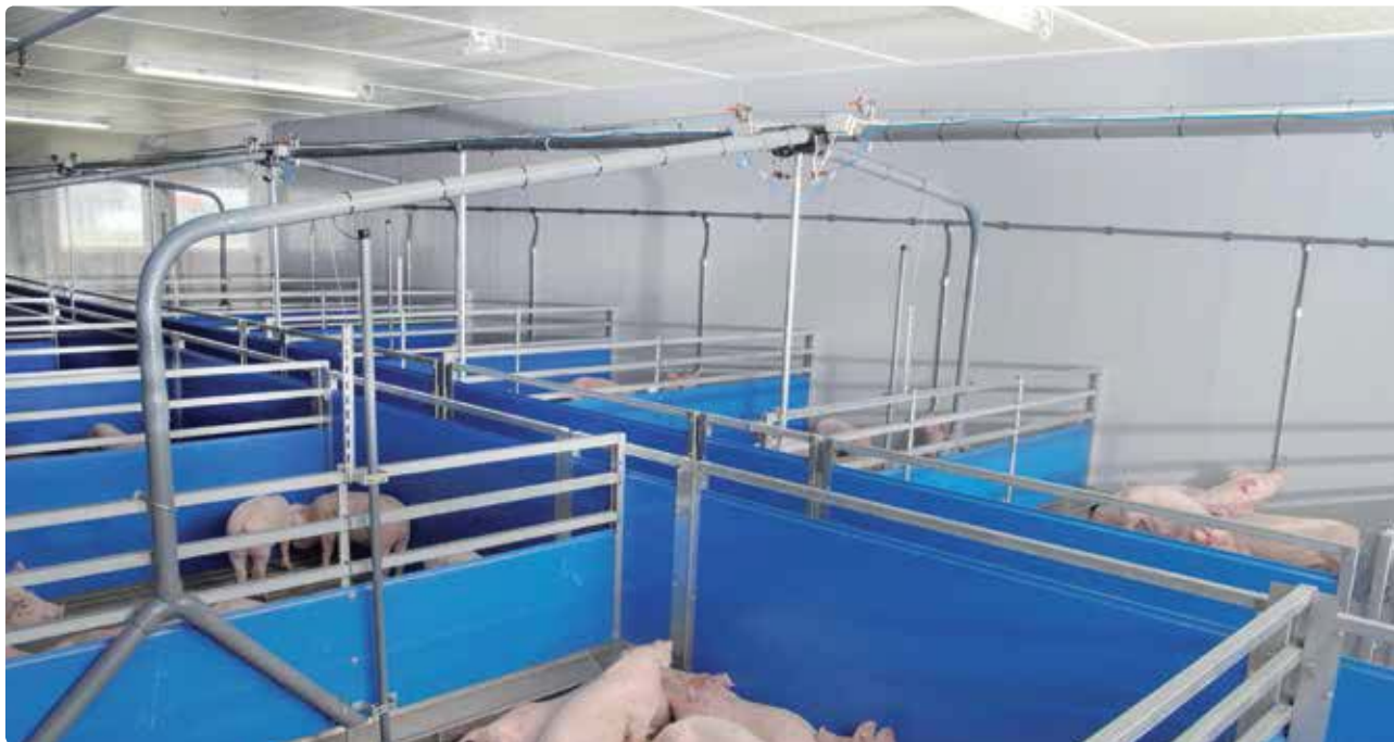
Feed line installed above the walkway.
