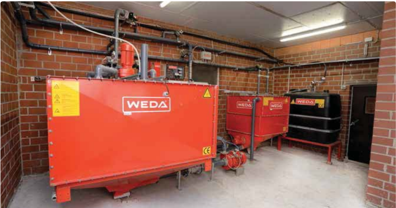
In case of very large distances between feed preparation and animal location, feed provision takes place via satellite preparation room.
